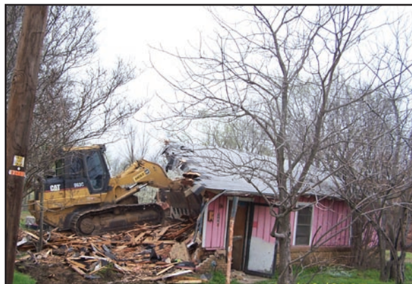
The City of Kaufman recently contracted for the demolition of a substandard house located at 1205 East First North.
